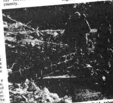
FLASHBACK to November 27: Mayfield telephone exchange is reduced to a pile of rubble.
